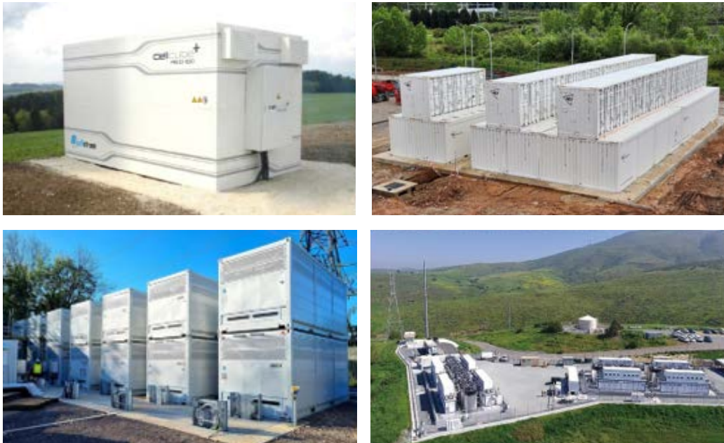
Fig 8: VFB projects in Europe and North America (top left: system in Lietenegg, top right: system in Spain, bottom left: system in Oxford Energy Superhub, bottom right: system in San Diego).
