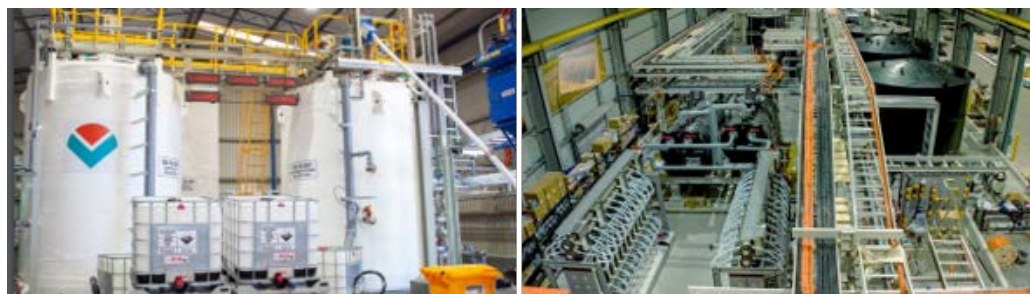
Fig 9: Vanadium electrolyte manufacturing facilities in Western Australia (left) and Queensland (right).
